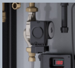
High Flow Recovery Pump
